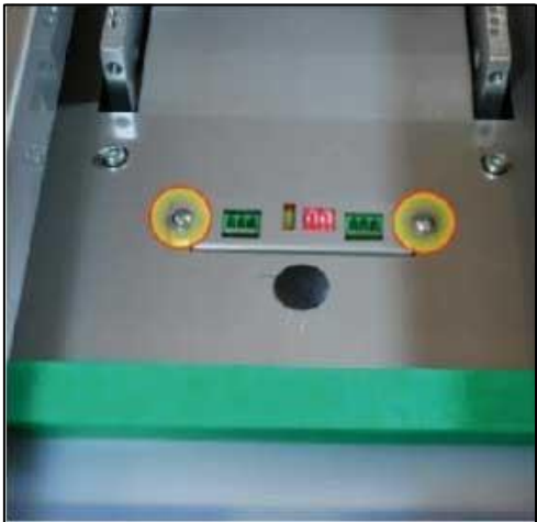
Figure 6-7: LED Controller (installed)
